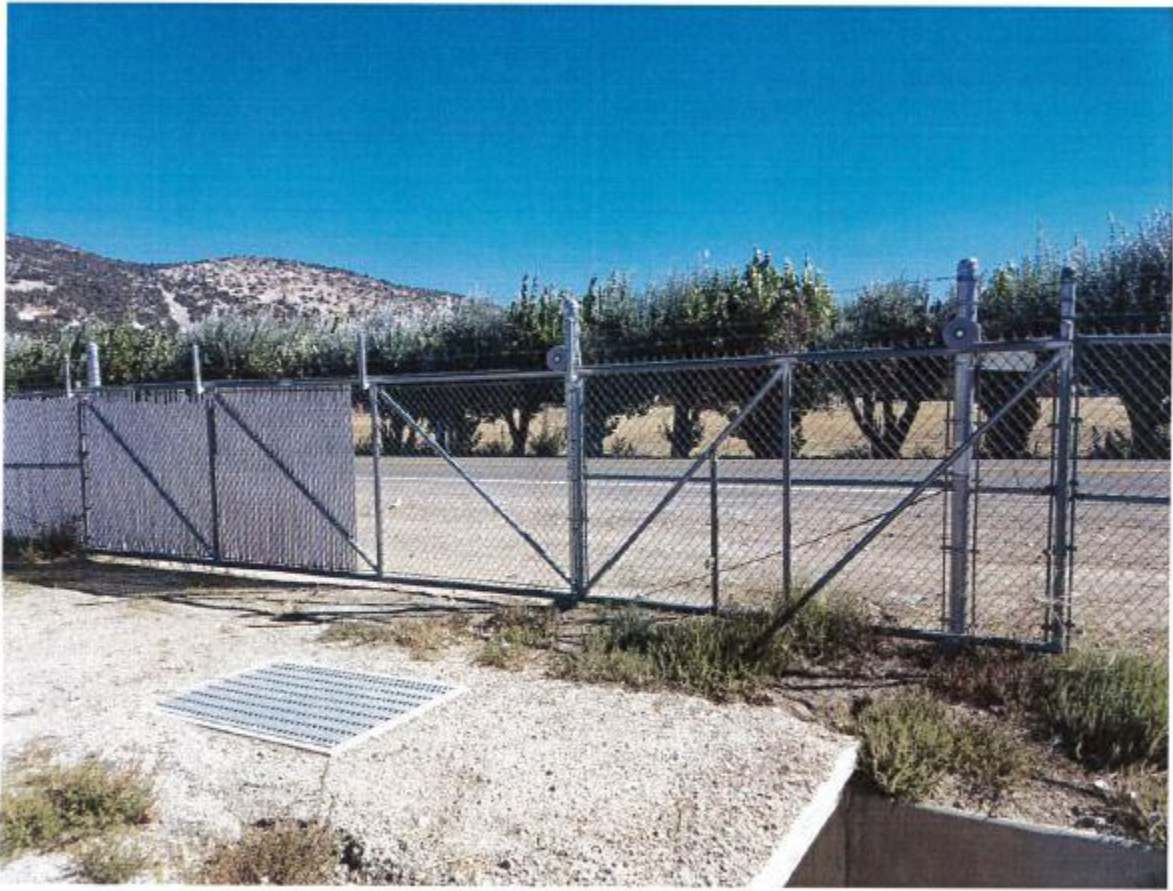
Manual cantilever gate currently installed on airport
